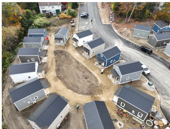
Cottages at Back River in Dover, as seen in 2023 while under construction. Photo: Tom Morgan
